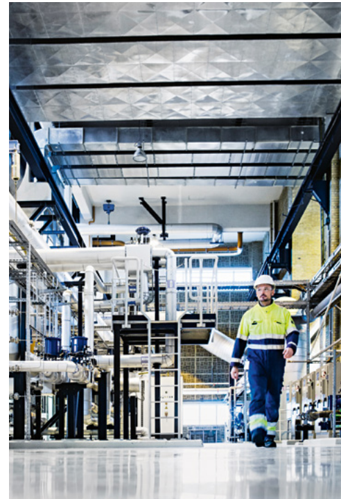
An employee at Öresundsverket Power Plant in Sweden.
